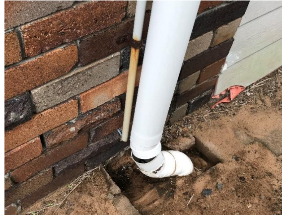
Photograph 5: Fault opening in PVC stormwater down pipe along southern external wall of site house, facing north east
