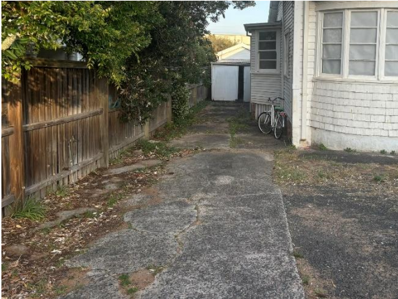
Photograph 5: Cracking within front driveway concrete pavement (No.140), facing west
