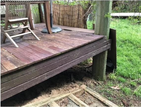
Photograph 4: Timber deck within rear of site, with rotation/rotting of timber planks and minor settlement evident, facing south west
