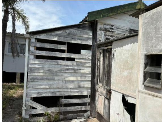
Photograph 6: Rear of garage structure (No.140) in a dilapidated condition, facing east
