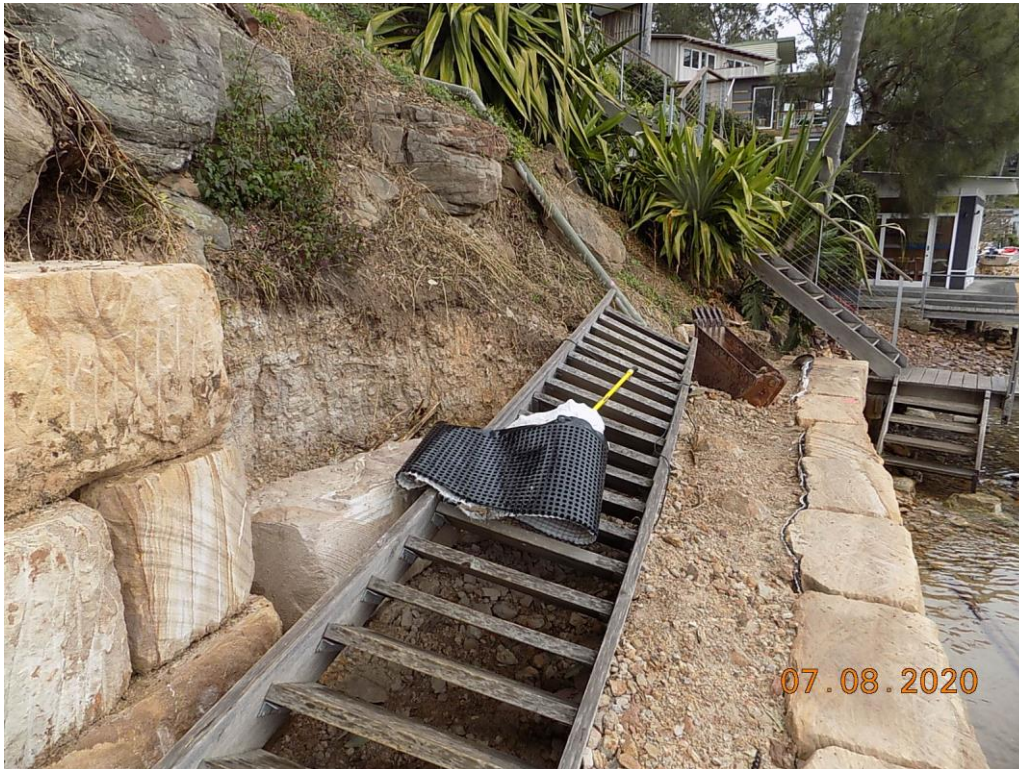
Photo 9: This portion of the slope is under construction as part of a separate DA.
