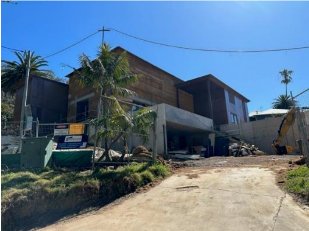
Figure 18 - Photograph of the dwelling house under construction at 2 – 4 Bilgola Avenue with a 3 storey presentation and 9.5 metre maximum building height.
