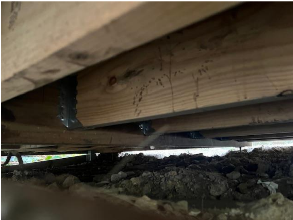
Photo 4: Existing conditions of joist hangers & bearer
