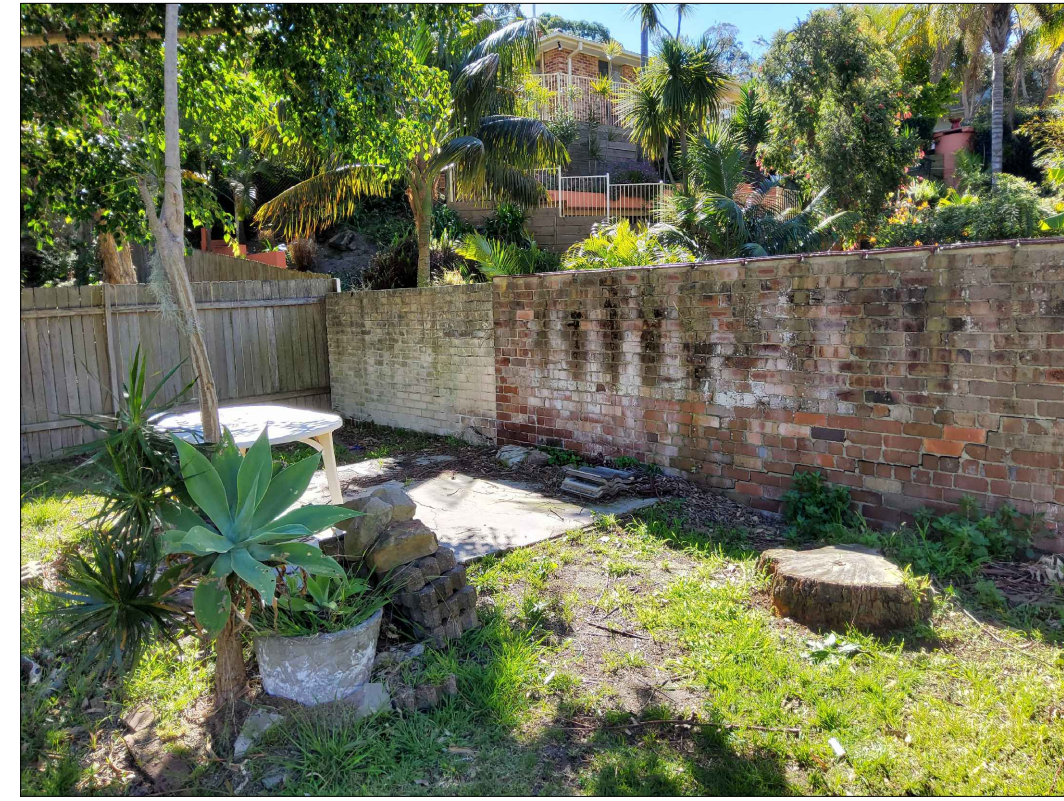
NORTHERN BOUNDARY NEAR COUNCIL DRAINAGE ASSET. MASONRY WALL TO BE RETAINED AND REPAIRED
