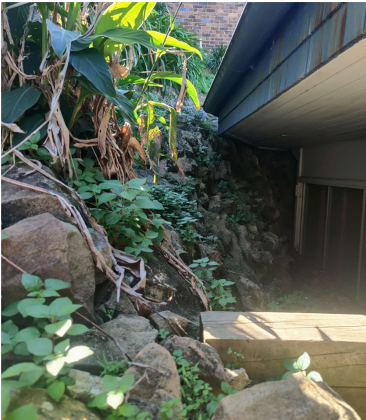
Plate 5 - Hazard D1a and D1b and D3 (2 Photographs)
