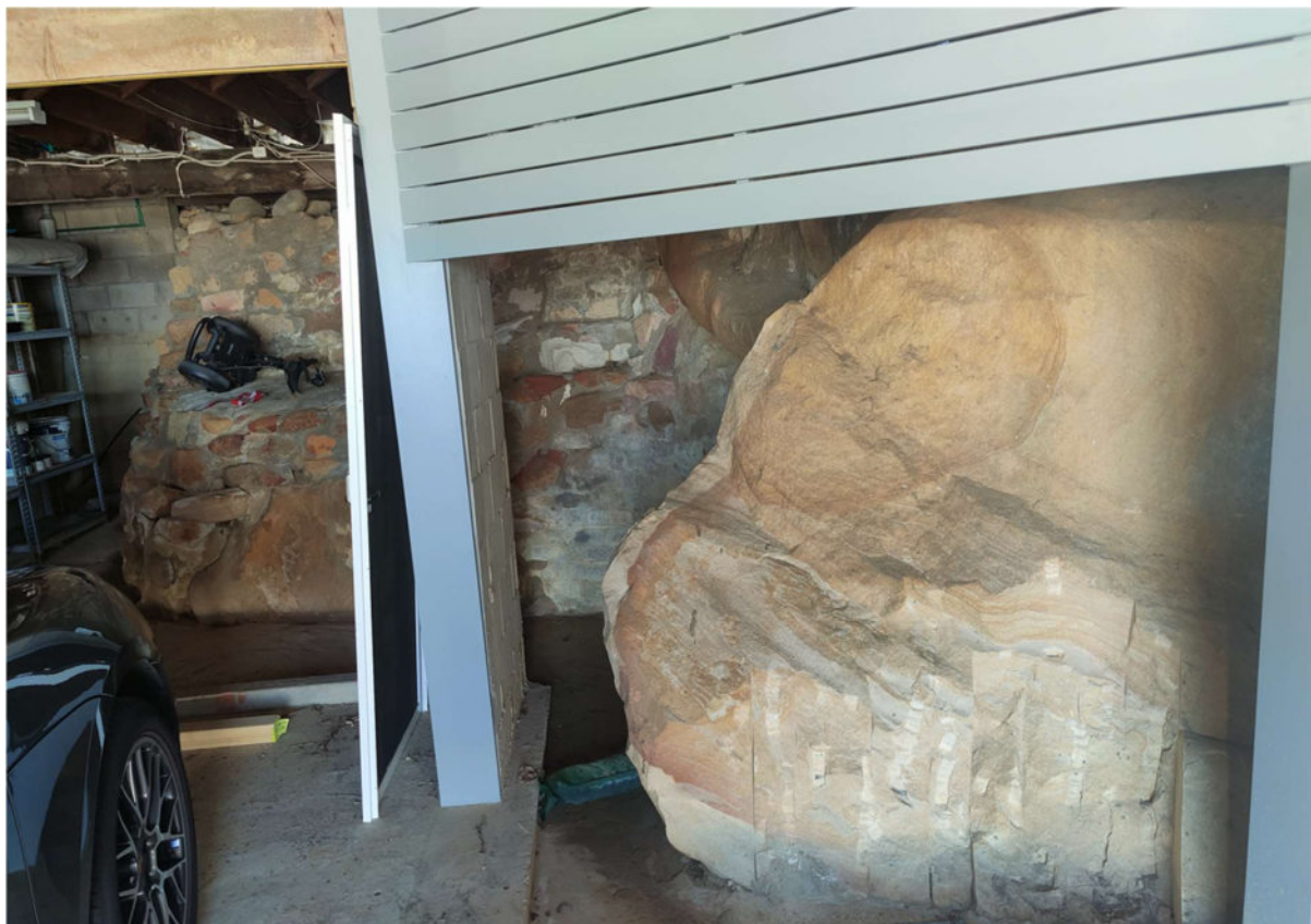
Plate 7 - Hazard D1b and D3 and Large Boulders in garage (1 Photograph)
