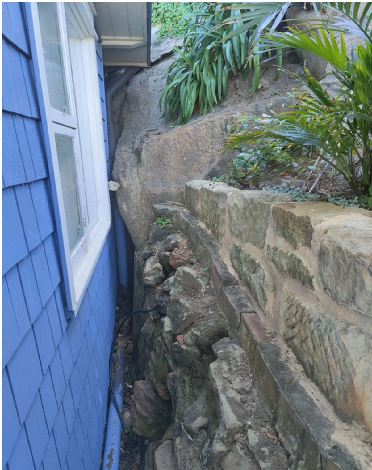
Plate 6 - Hazard D1b and Large Boulders on Northern Boundary (1 Photograph)
