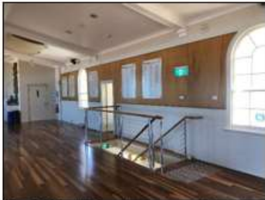
Figure 86. Main Club Room. Note staircase leading up from ground floor. (Source: Heritage 21, 23.05.18)
