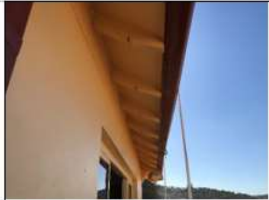
Figure 105. Note timber batons along roof line of original building in the centre. (Source: Heritage 21, 23.05.18)
