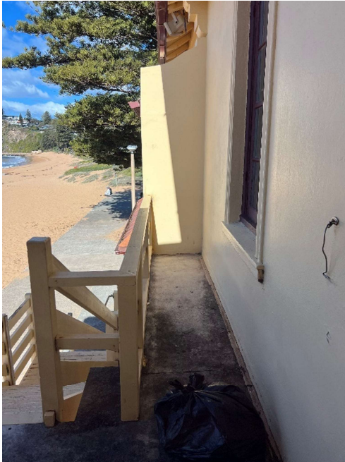
Figure 46 - View of the original first-floor ledge with the later timber stair leading to the walkway in front of the clubhouse. (Source: NBRS)
