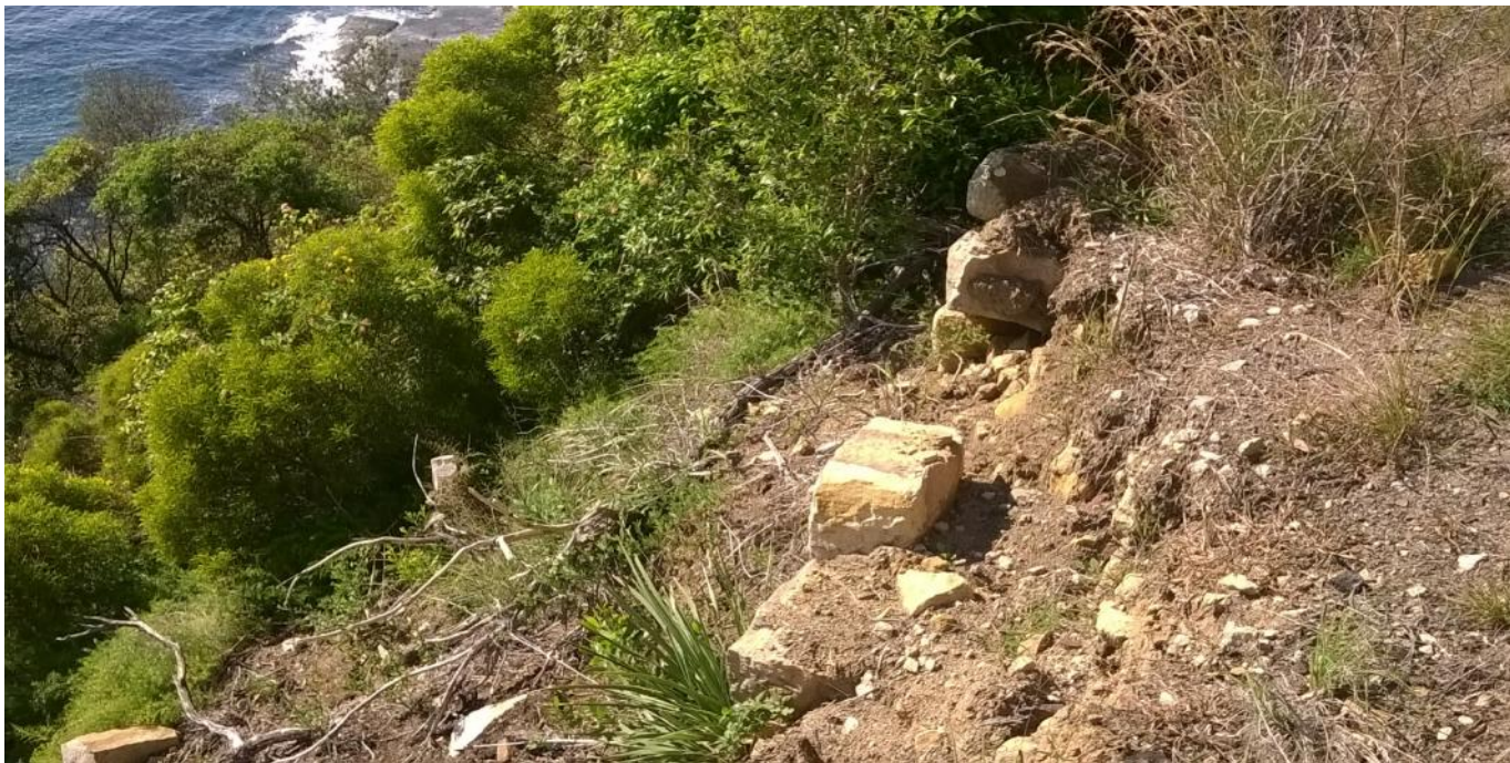
Photo 3: View of a failed retaining wall at the Whale Beach Site 1
