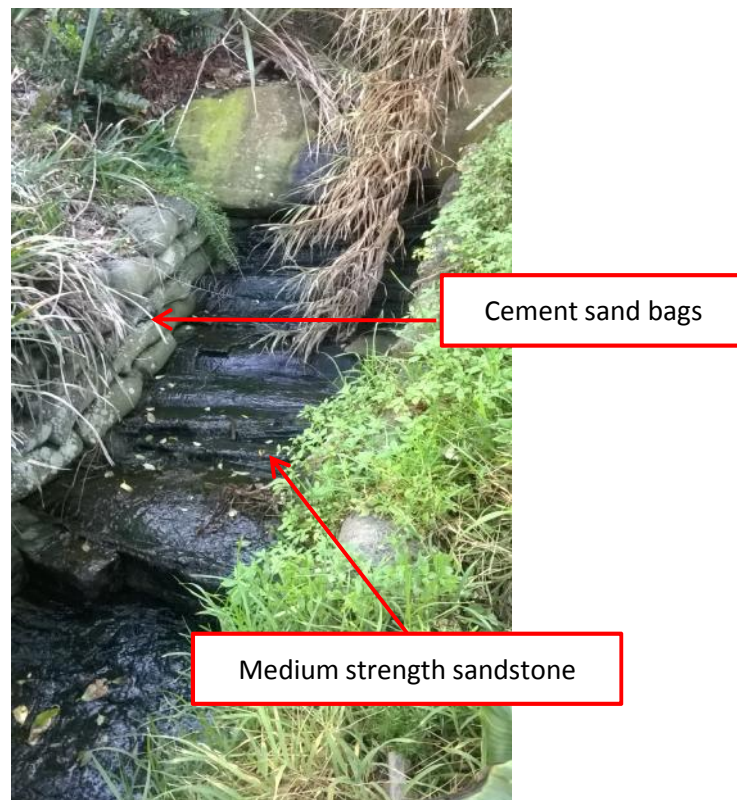
Photo 7: View of a failed retaining wall at Bilgola Beach Site 2
