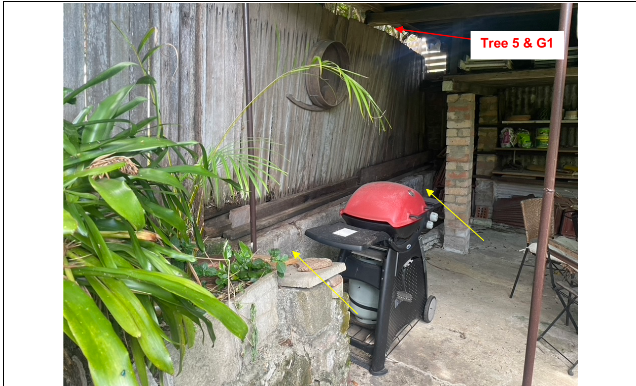
Photo 2: Looking Southwest from within the site towards the rear boundary, showing the existing boundary retaining wall (yellow arrows). The existing boundary retaining wall appears to be restricting root from tree 5 and G1, therefore, tree 5 and G1 will not be impacted by the proposed works within the site. Tree 5 and G1 are located behind the boundary fence within the adjoining property and are not visible in this photo.
