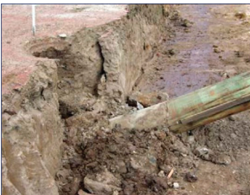
Excavation causing pole collapse
