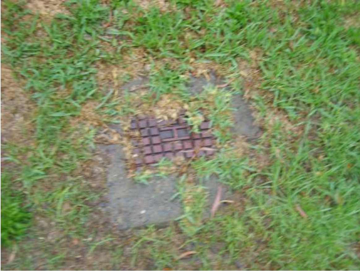
Photo 2 – Indicates the reticulated mains pressure fire hydrant located outside No.19 Sherwood Crescent (Steve Brooks 2020).
