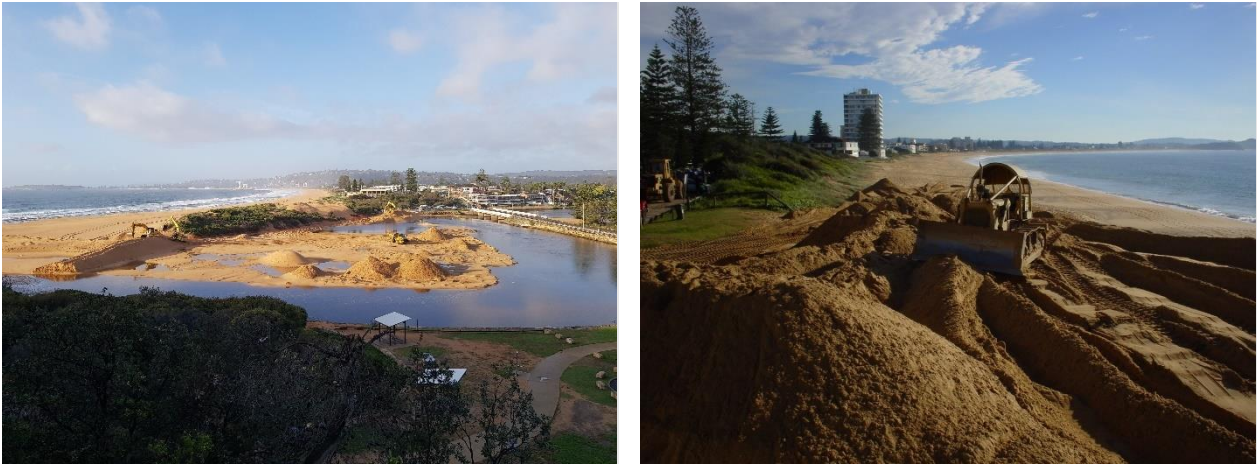
Figure 2-16: Excavators removing the entrance shoals (left), Unloading and regrading of sand for beach replenishment (right)
