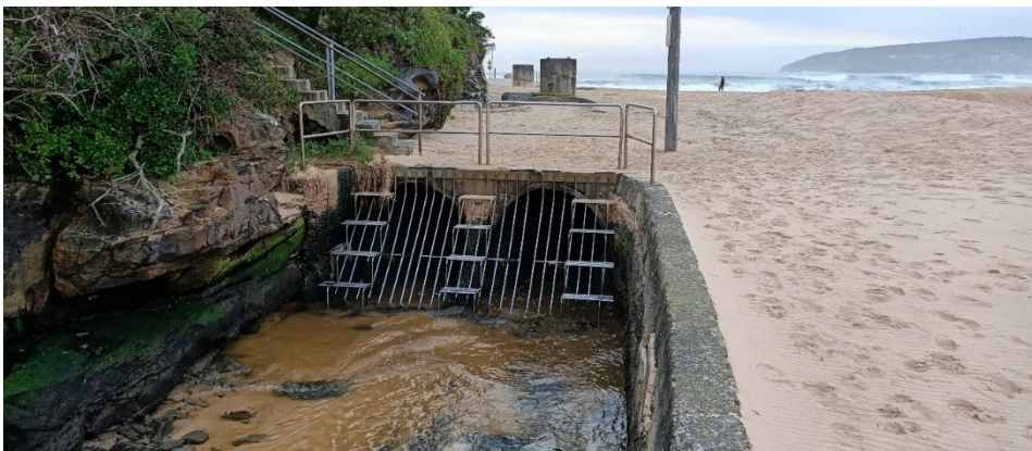
Figure 6-8: Existing low flow pipes at Manly Lagoon beneath the beach berm at Queenscliff Beach
