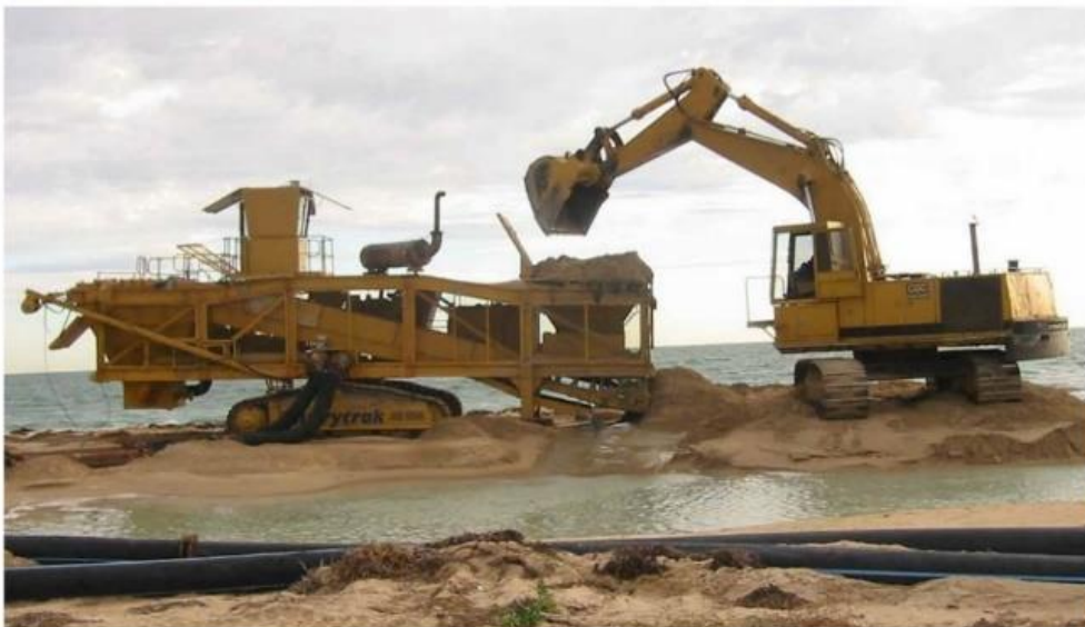
Figure 6-3: Slurrytrak system operating at Dawesville and Mandurah Inlets, Western Australia
