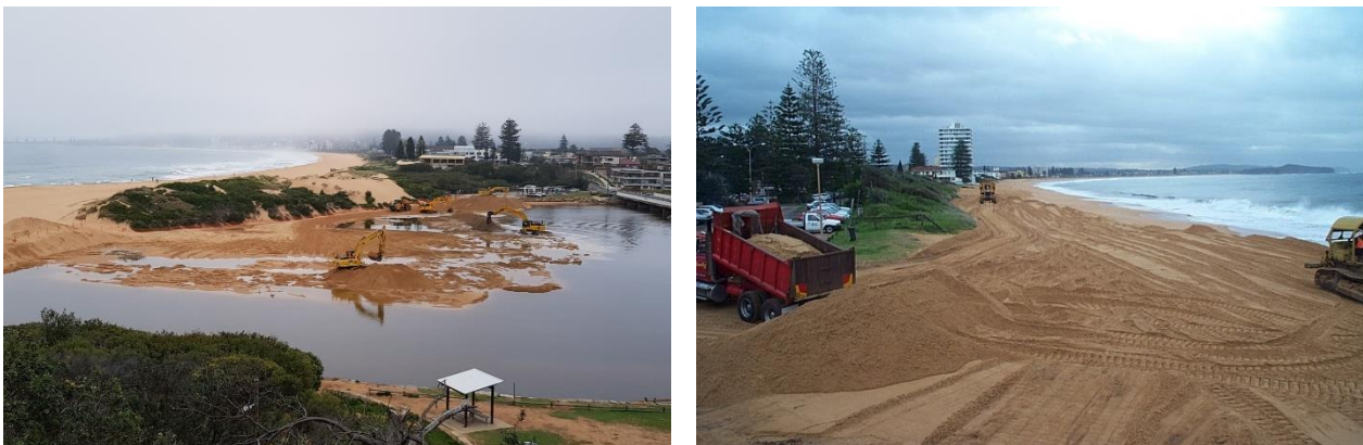
Figure 5-1: Excavators removing the entrance shoals (left), Unloading and regrading of sand for beach replenishment (right)
