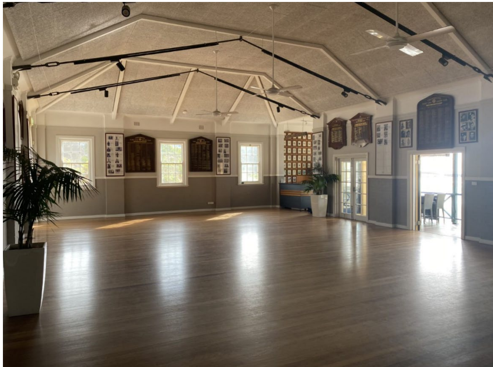
Figure 27: Interior of the surf club building (Level 2), view looking east (Source: NBRS, 1 February 2023)
