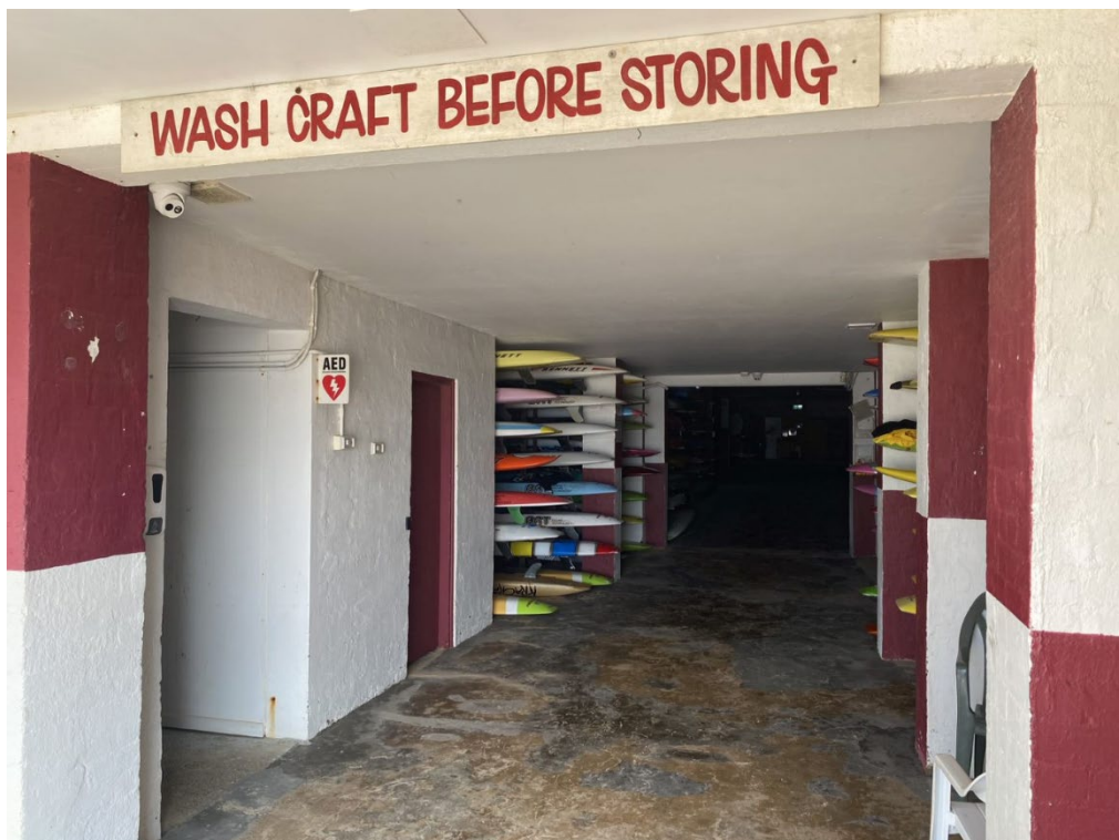
Figure 29: Basement of the original surf club building (Level 1), view looking west (Source: NBRS, 1 February 2023)
