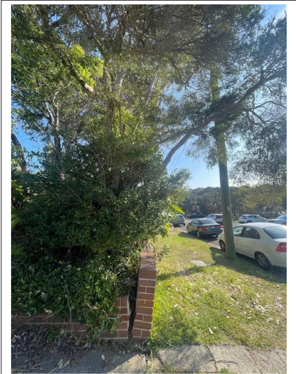
Photo A: The front boundary retaining wall is in a state of disrepair.
