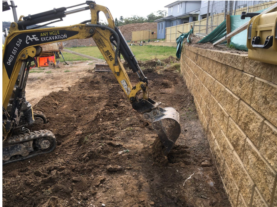
Photo 1: Photo shows excavation works to expose the part of the footing of the existing wall for full engineering analysis at 79 Lorikeet Grove, Warriewood
