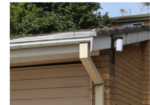
3. FASCIA, GUTTER - TO MATCH EXISTING DOVER WHITE OR SIM. DOWN PIPE - CLASSIC CREAM OR SIM.
