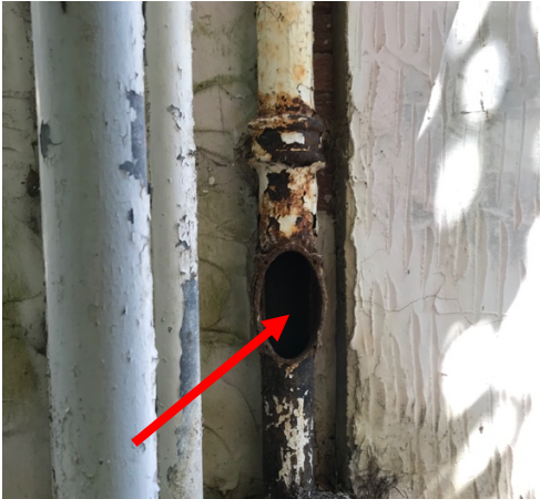
Disused drain pipe opening in the north eastern area on the house.
