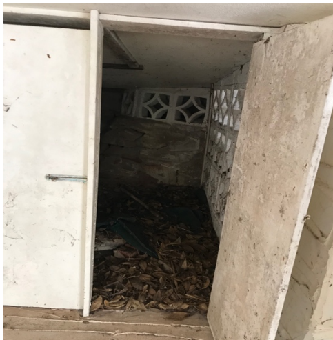
Cave like storage area on the bottom floor on the western side of the property (door was closed)
