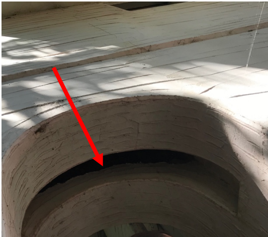
Cavernous opening in the north eastern area of the house.
