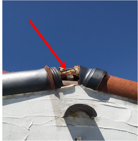
Opening in the roof tiles in the north facing wall of the house.
