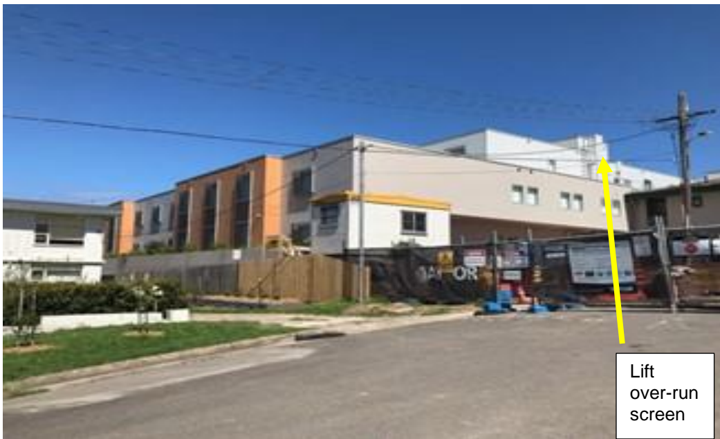
View from Patey Street looking south-east at the end of the cul-de-sac. The lift over-run and screen are visible.
