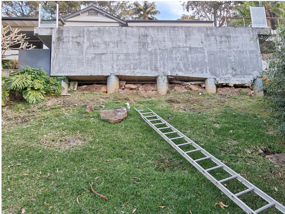
Image 9. Swimming pool shell to be screened and retaining wall to be constructed to facilitate the level turf area.
