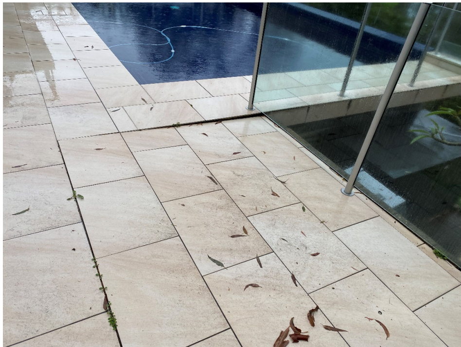
Image 3. Section of slumped tiling to be replaced.
