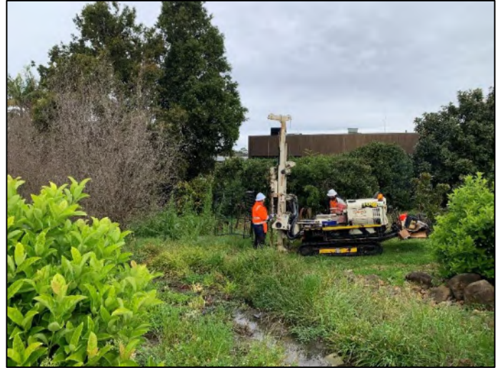
Plate 8 – Drill rig set up near the storm water retention dam at south-west side of the site.
