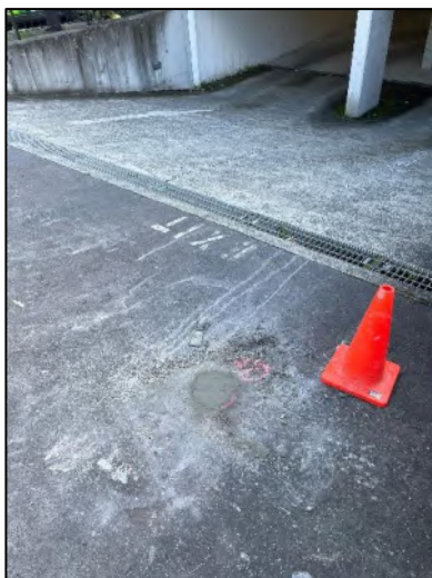
Plate 11 – View of boreholes refilled with concrete after concrete cutting and soil sampling.
