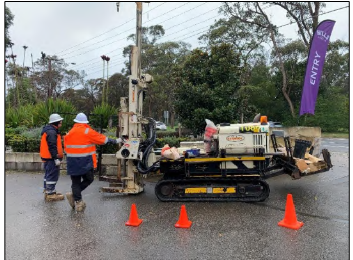
Plate 2 – Drill rig set up near to the entrance of the site from Mona Vale road in the south-east side.
