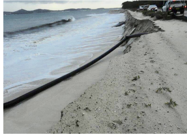
Damage to Jimmys Beach sand transfer system by large swell in 2019 (Source: Newcastle Herald, 5 June 2019)
