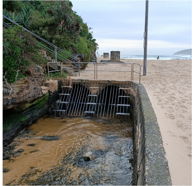
Existing low flow pipes at Manly Lagoon beneath the beach berm at Queenscliff Beach
