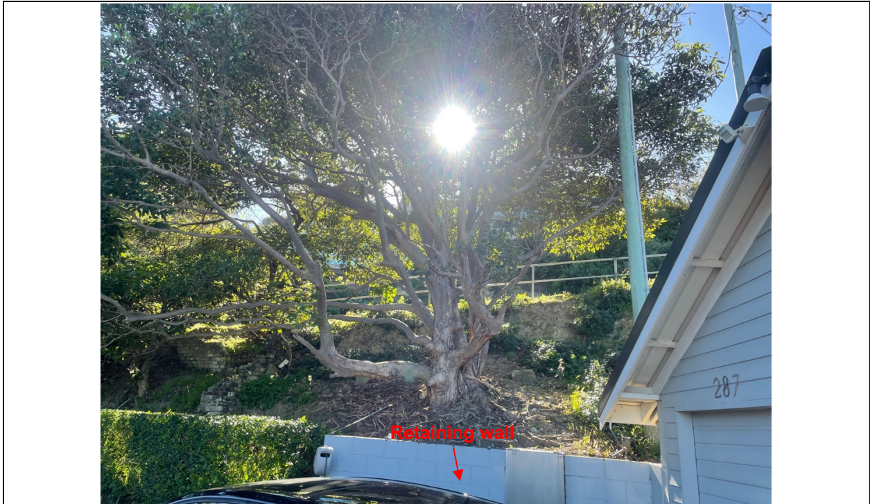
Photo 1: Looking towards tree 2 from within the site, showing the existing retaining wall which appears to be restricting significant root growth towards the area of the proposed works.
