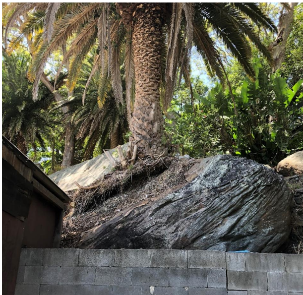
Photograph-3: Wash out under roots of palm tree, looking east
