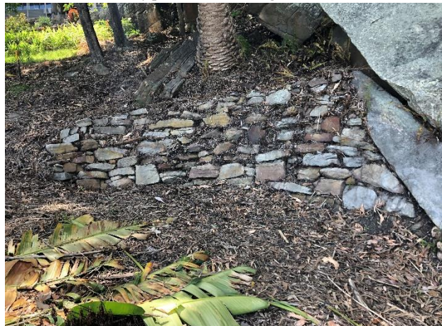
Photograph-6: Retaining wall to the north of sandstone boulder along the eastern edge of the middle-terraced region, looking east
