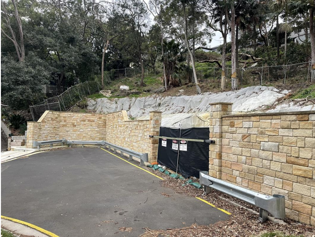
Fig 2: View of the Bellara Avenue eastern cul-de-sac and driveway entry to the subject sites (via 32 Bellara Avenue), looking north-east
