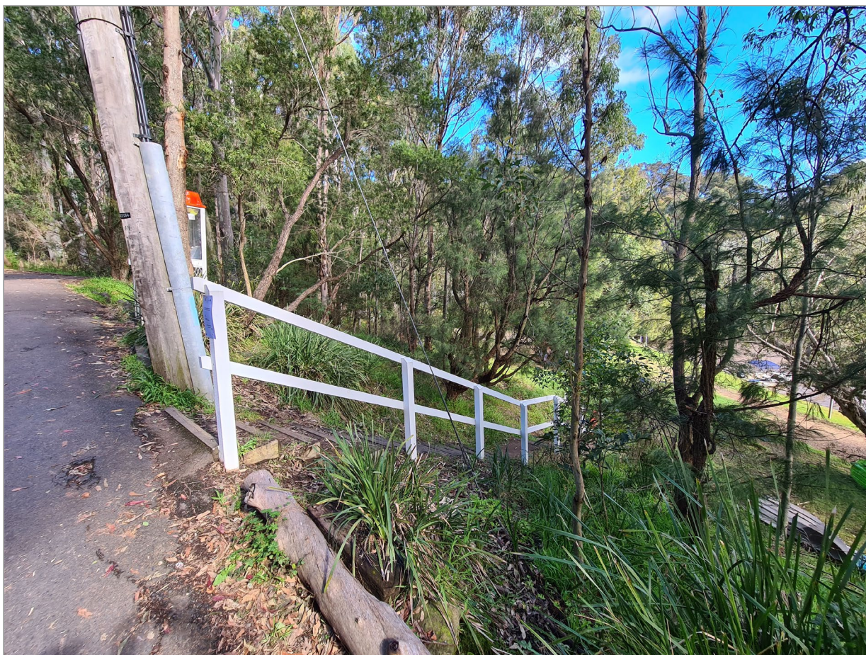
Photograph 6: Commence of low hazard to the south-west
