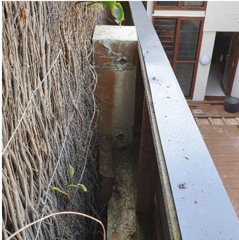
Photograph-8: Brick retaining wall along the north boundary. View looking down east.
