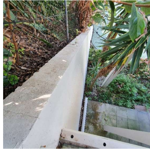
Photograph-7: Brick retaining wall along the north boundary. View looking down east.
