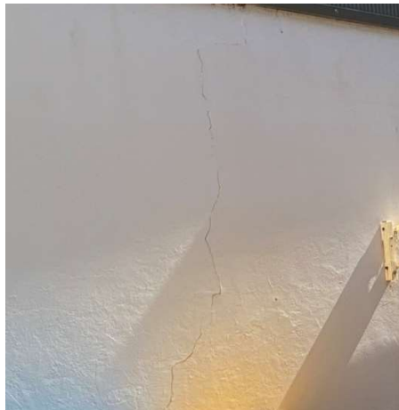
Photograph-10: Cracking within the retaining wall. View looking west.
