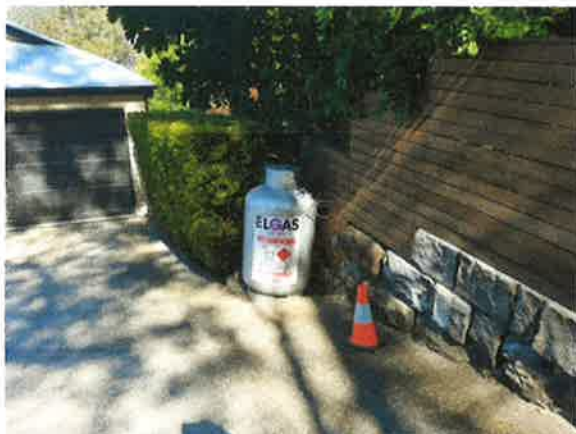
Existing gas supply
