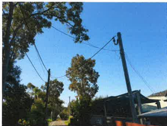
Existing electrical supply
