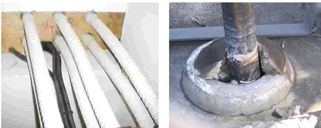
Figure 19 – Asbestos cable tape in substation and broken NC compound
