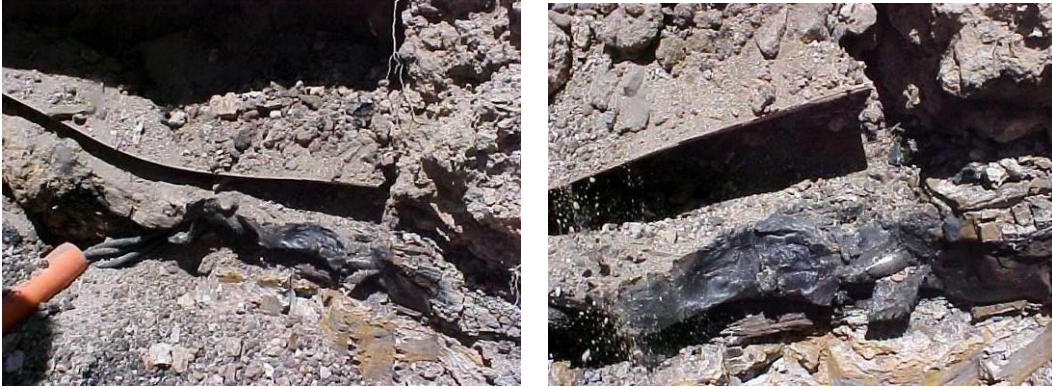
Figure 15 – Damaged bitumen encased cable with polymeric cable cover
