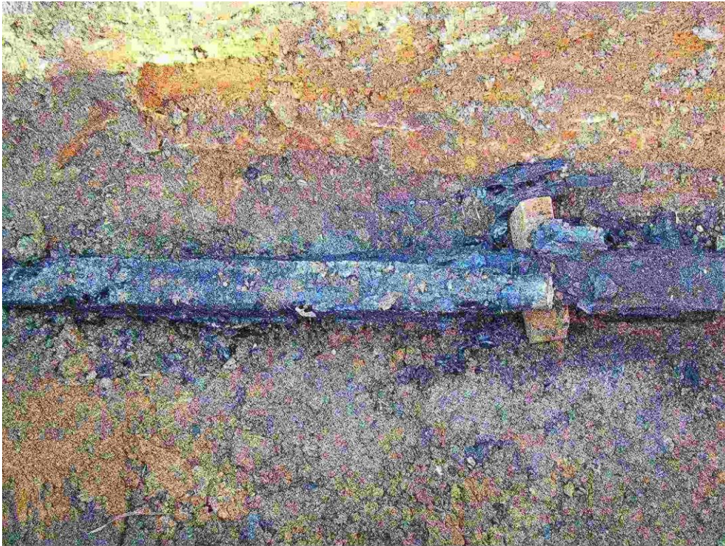
Figure 16 – Damaged bitumen encased cable
