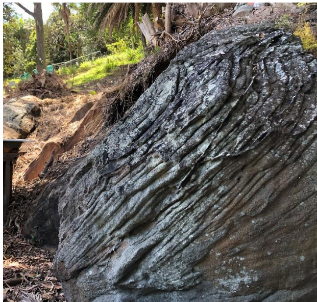
Photograph-4: Sandstone boulder and wash out under roots of palm tree, looking north east
