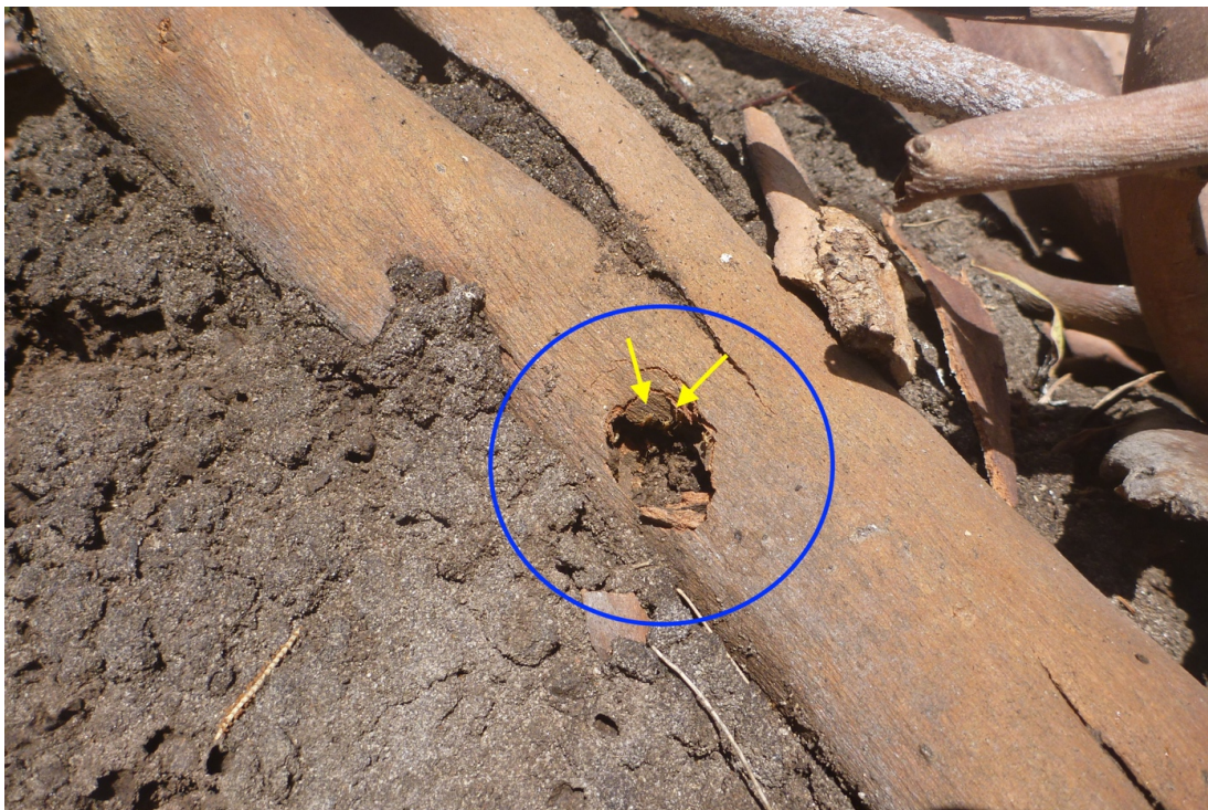
Figure 15 - Blue circle shows hole from probe to determine if nest is active, yellow arrow shows active termites
