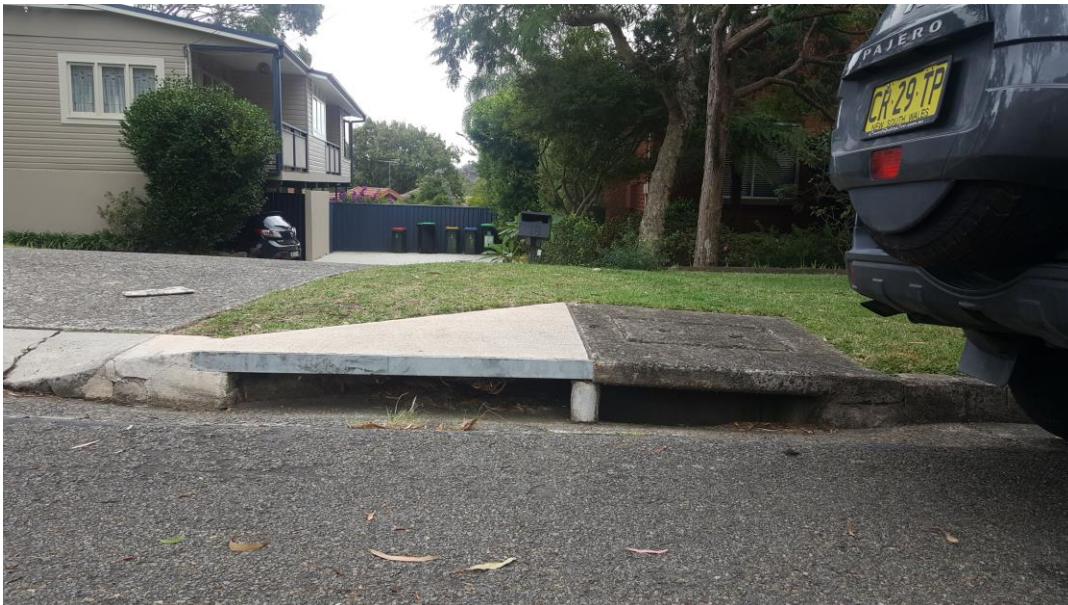
Figure 3. Existing on-grade pit (no grate) at 16/18 Dareen Street – front view
