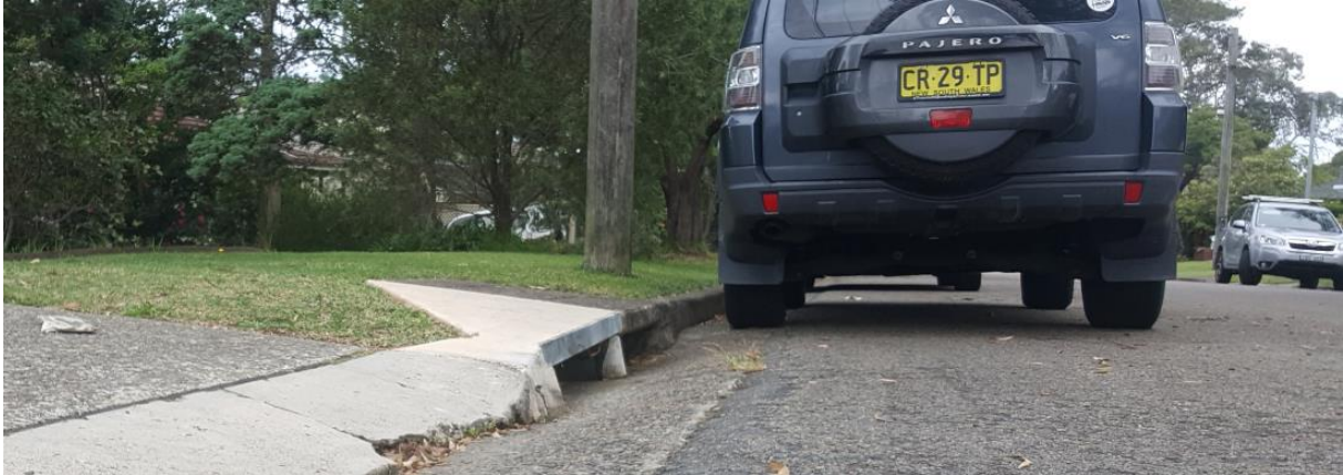
Figure 3. Existing on-grade pit (no grate) at 16/18 Dareen Street - side view with crest - photo looking downstream.
