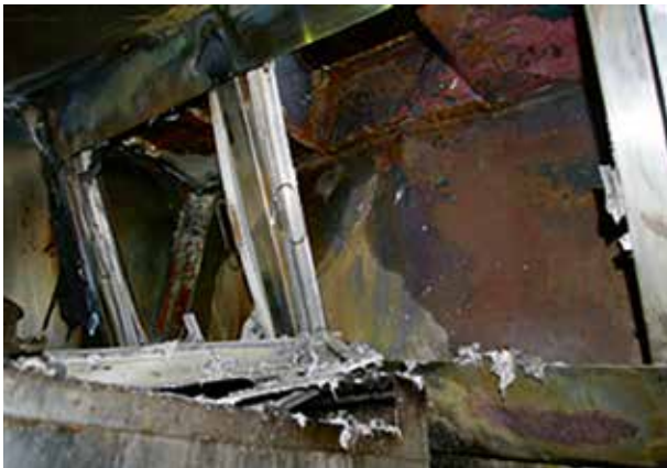
Figure 8: Burnt grease filters.
