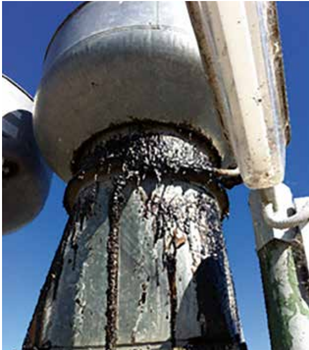
Figure 15: Grease leaking from ducts and pooling on roof.
