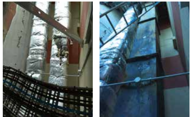
Figure 17: Insulation prevented fire breaking out of this exhaust duct.
