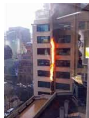
Figure 18: Fire rapidly spreading up a vertical kitchen exhaust duct.
