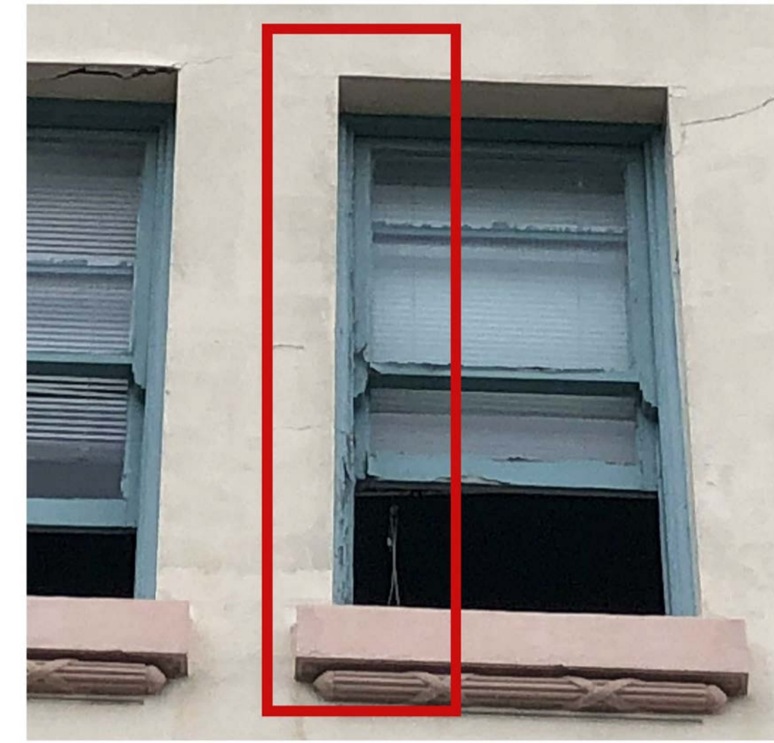
Open up render over all windows and investigate corrosion of lintels. Replace or rectify lintels to structural engineer and heritage architect's advice and reapply render to match original detail
