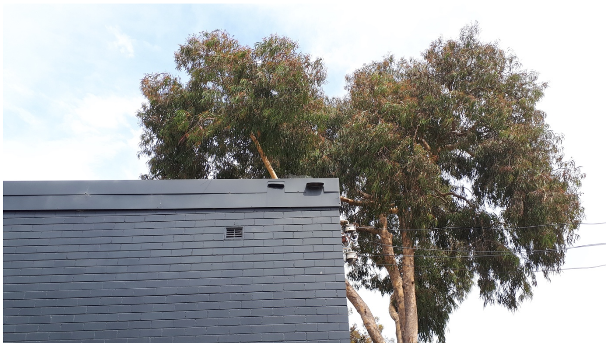
Photo 4: Extent of canopy overhanging building.
