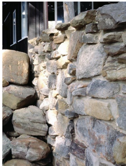
Garden Walls: Irregular Garden walls.
