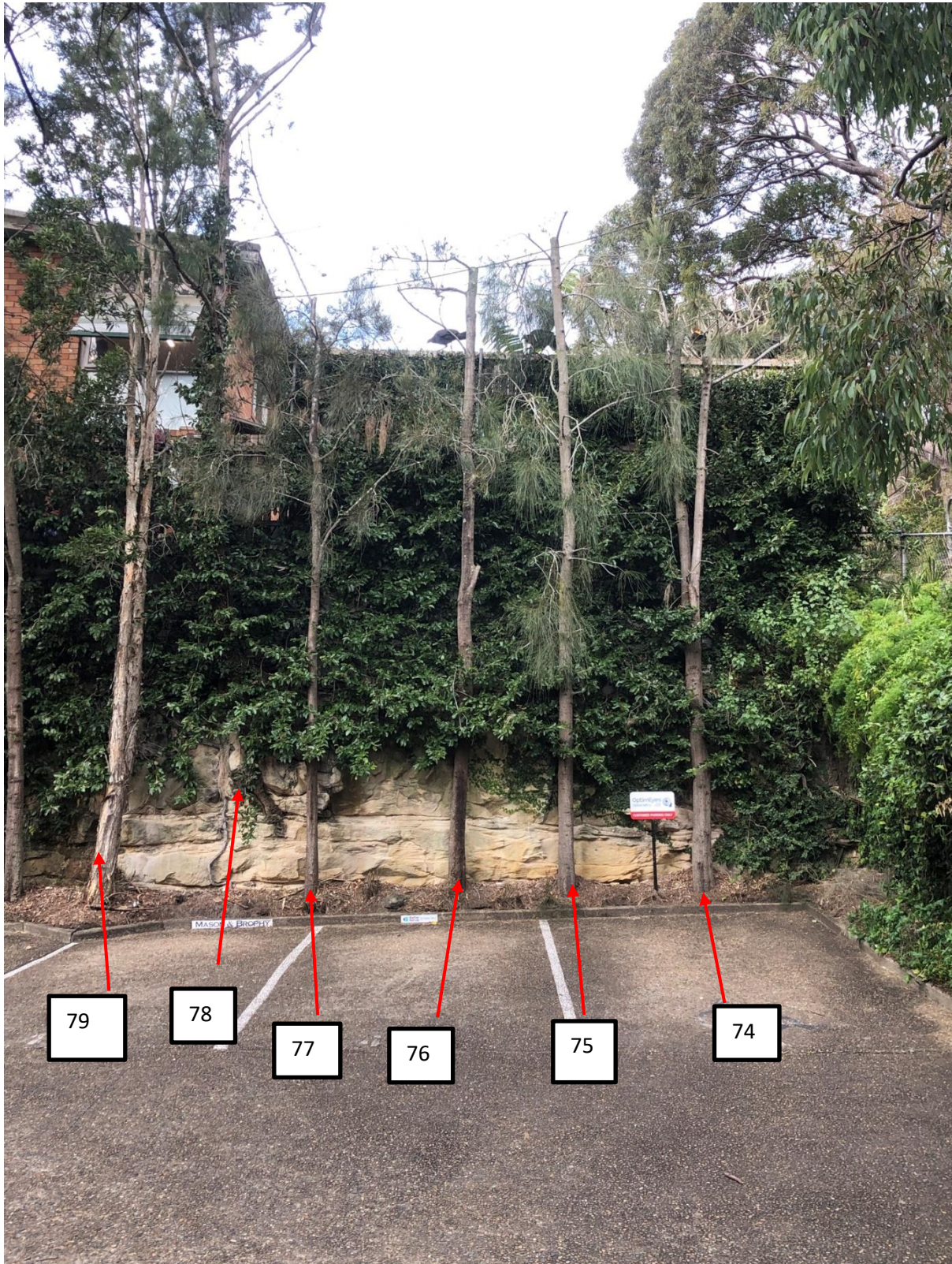
Trees 74 to 79 Trees 74, 75 76 77 have been lopped. Tree78 is growing out of rockface
