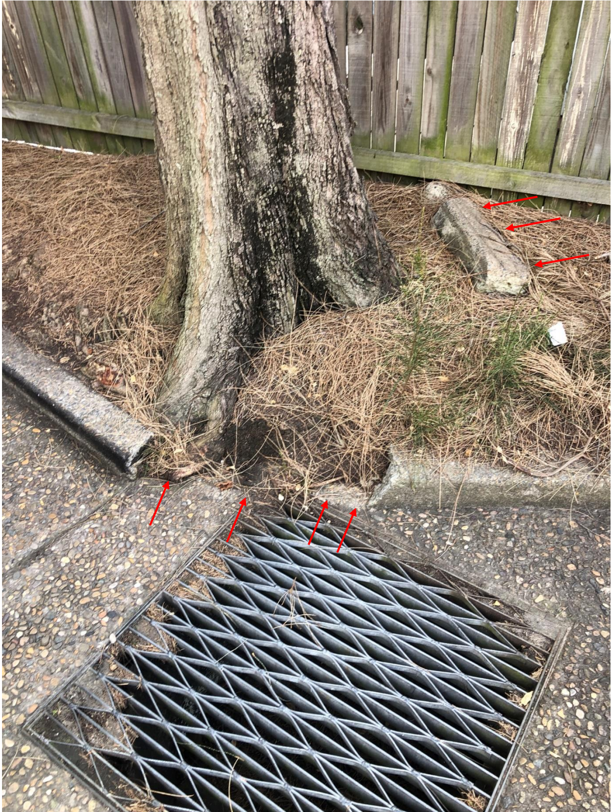
Tree 55 - Casuarina - has impacted concrete kerb
