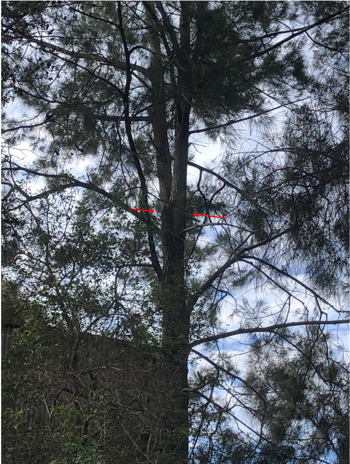
Tree 68 – Trunk inclusion at 7 metre mark
