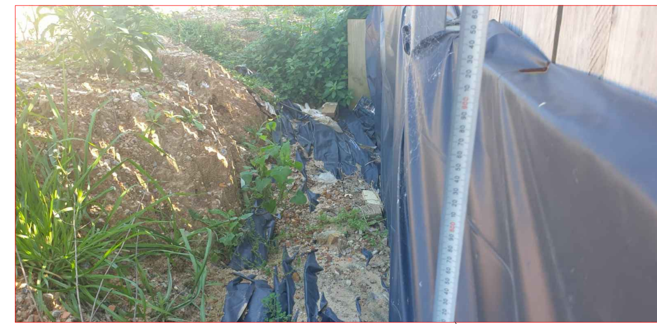
EXISTING CAVITY TO BE FILLED AND GRADED WITH AVAILABLE TOP SOIL (STOCKPILE) AFTER CLEANING THE DEBRIS.
