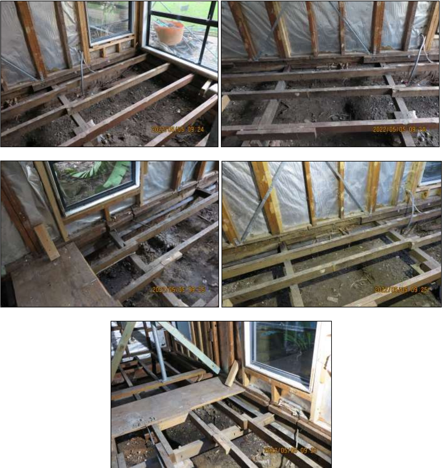
Figure 1: Above photographs confirm soil level conflicts, damaged built form & tree roots penetrating into & under the original floor.
