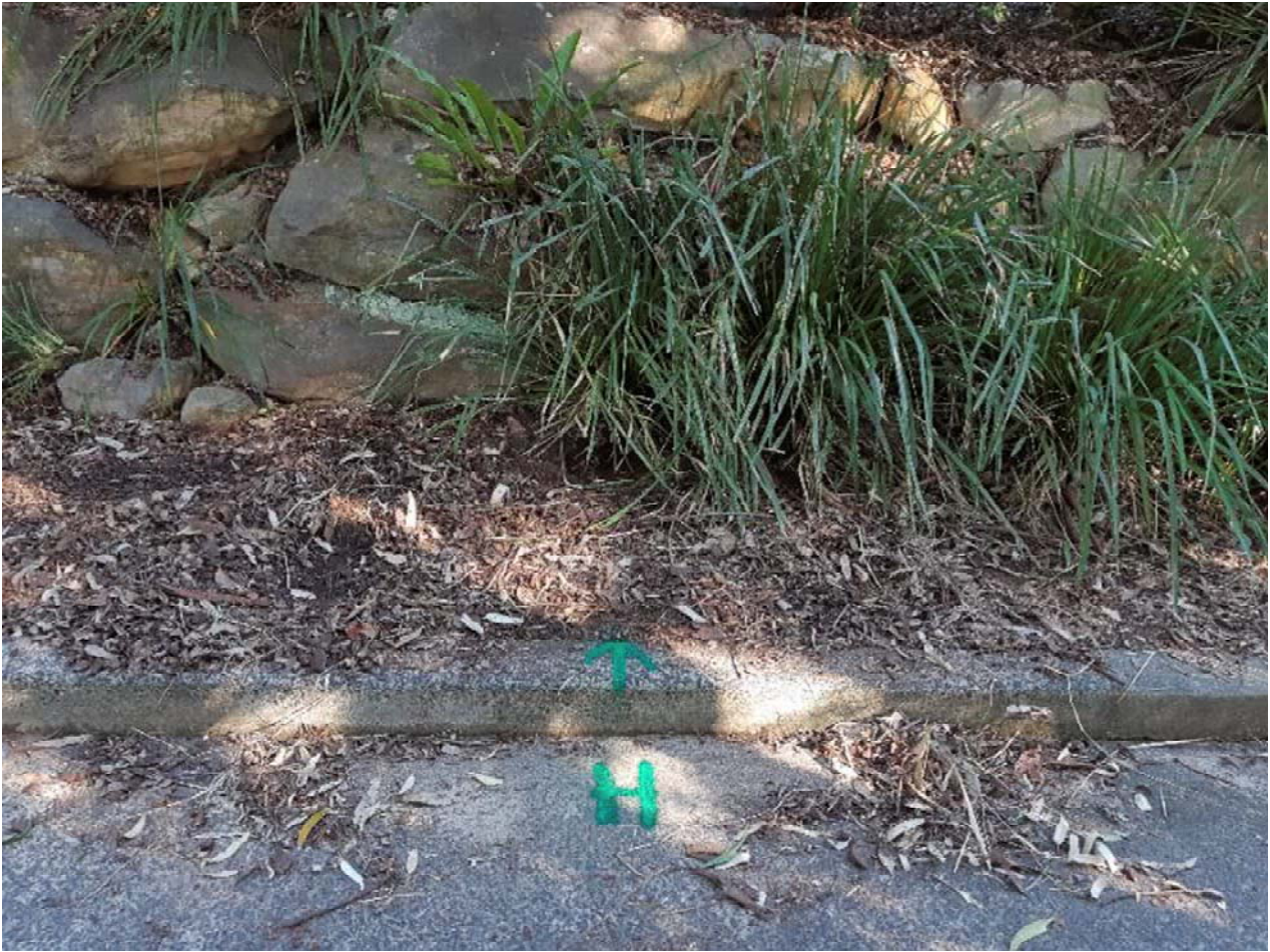
Buried hydrant on end of uPVC water
