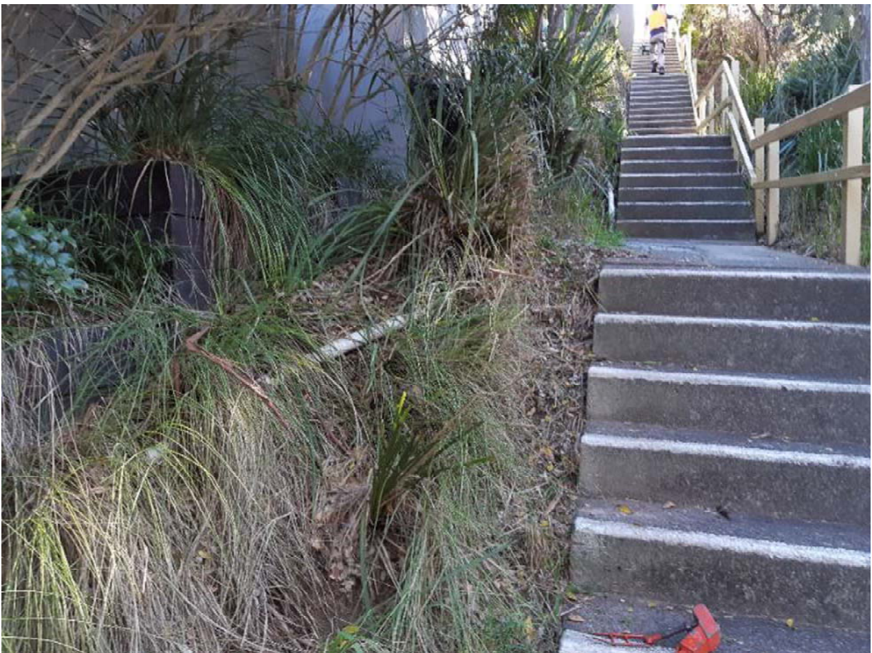
Comms in exposed conduit
