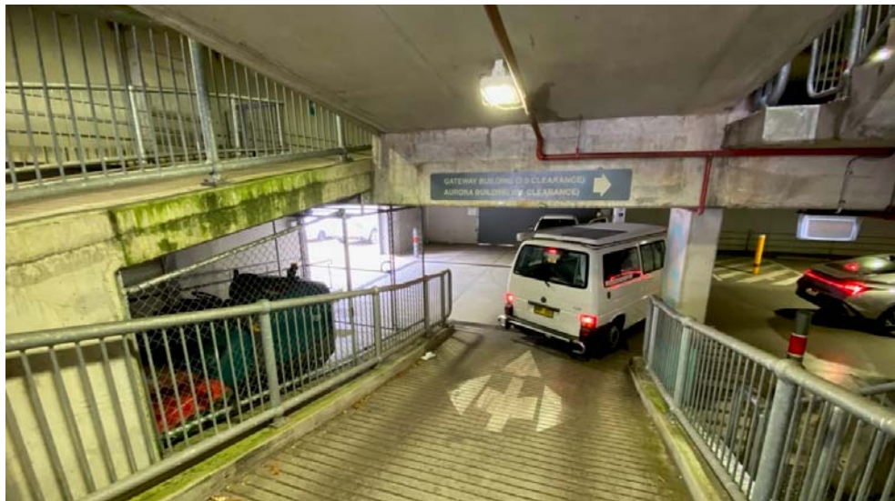
Photograph of the entry ramp to the access opening to 1749 Pittwater Road
