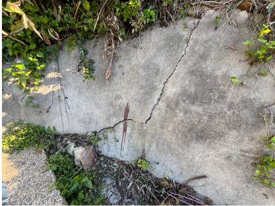
Photo 7: Cracking in the concrete wall on the western side of the pool
