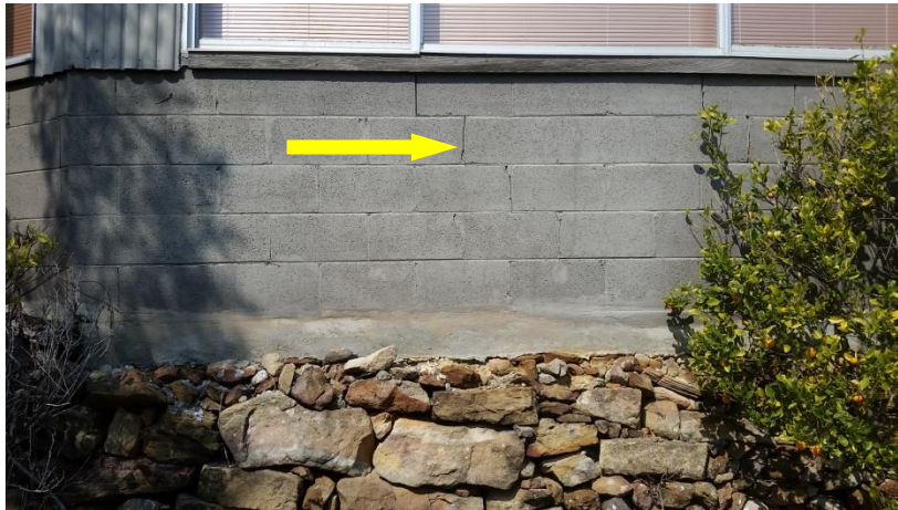
Photograph 4: Cracking observed in the lower section of the rear wall.
