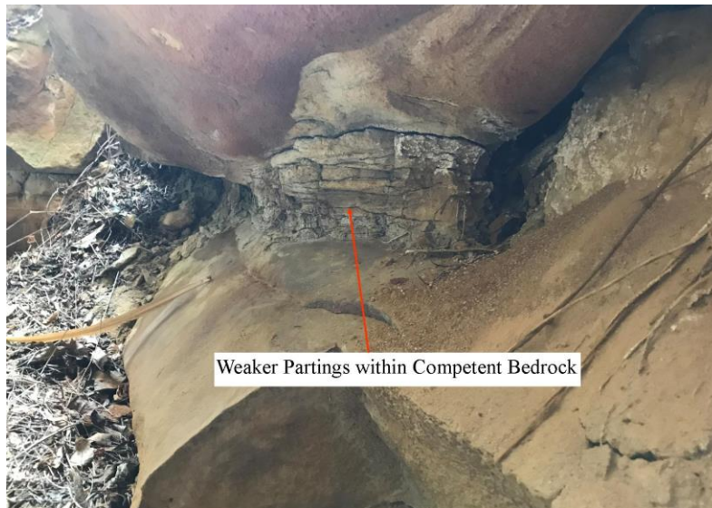
Photograph 12: Weak zones within bedrock
