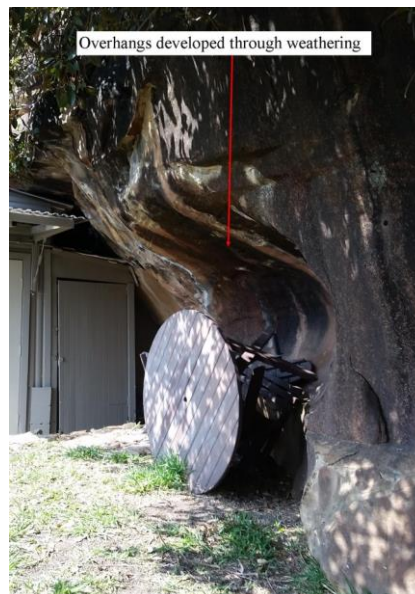
Photograph 8: Overhang/undercutting within the site.
