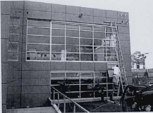
Rear-West Orientation: Note shade device pelmet above windows. Window at left not covered as this is the future lift shaft
