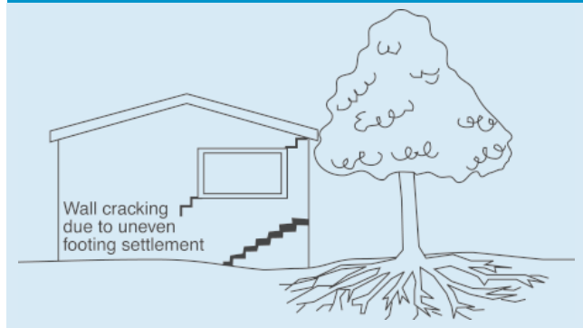
Trees can cause shrinkage and damage
