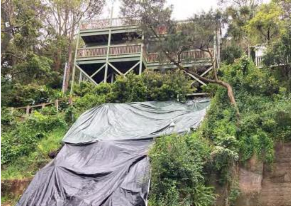
Figure 4: The site, looking north-west from Nareen Parade (after landslide)
