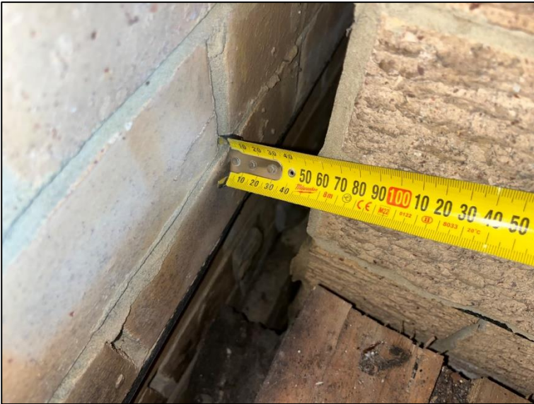
Photograph 3 – Separation between rear garage wall and partition wall
