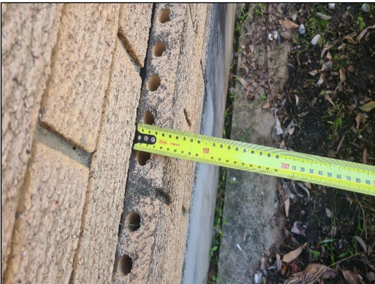
Photograph 8 – Displacement and rotation of masonry along damp proof course level
