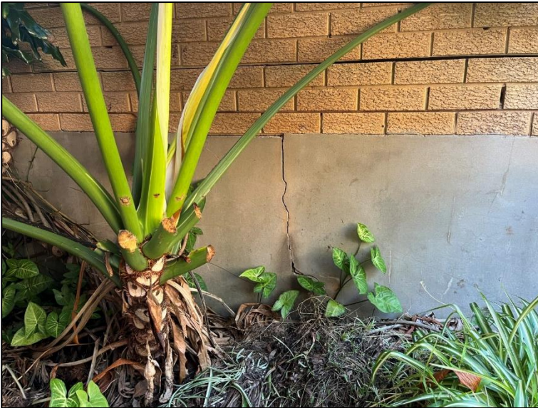
Photograph 7 – Vertical and horizontal cracking
