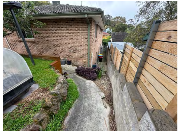
Photo 4: Masonry landscaping wall (right) showing an ~5-degree rotation from vertical.
