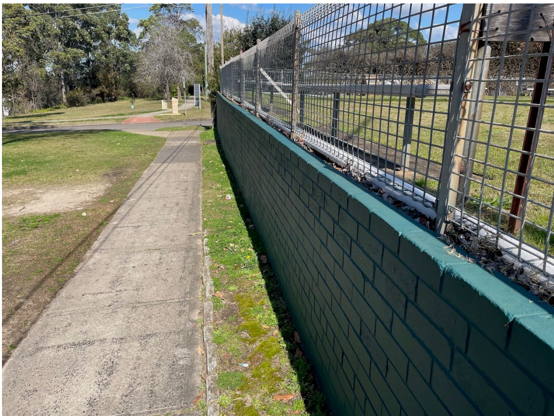
Plate 10 – Developed lean in highest section of the mortared brick retaining wall, viewed to south.
