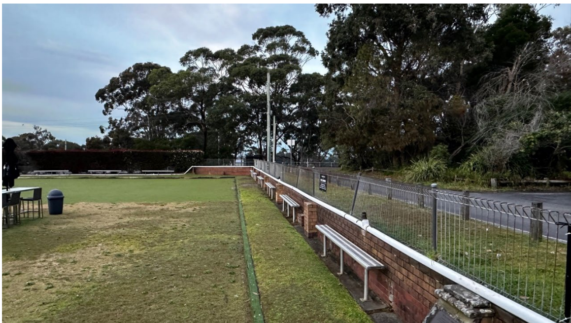
Plate 8 – View to the south, showing the low cut into the natural hillslope supported by a mortared brick retaining wall.
