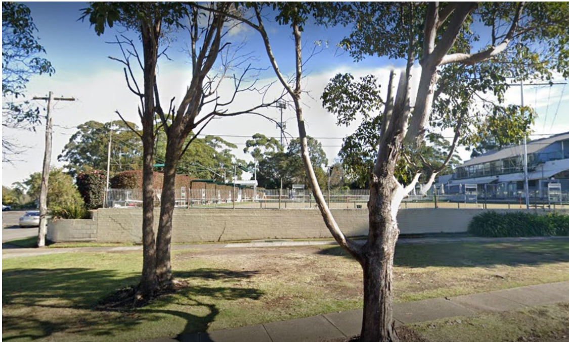
Plate 9 – Google Maps view of the mortared brick retaining wall at the southeastern corner of the site, prior to painting, detailing existing cracking.
