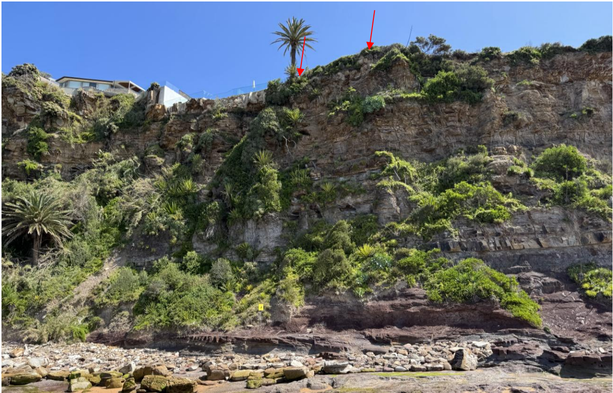
Figure 3: View of cliff face at site (approximately between arrows) from rock platform on 3 October 2024, facing SW to WSW
