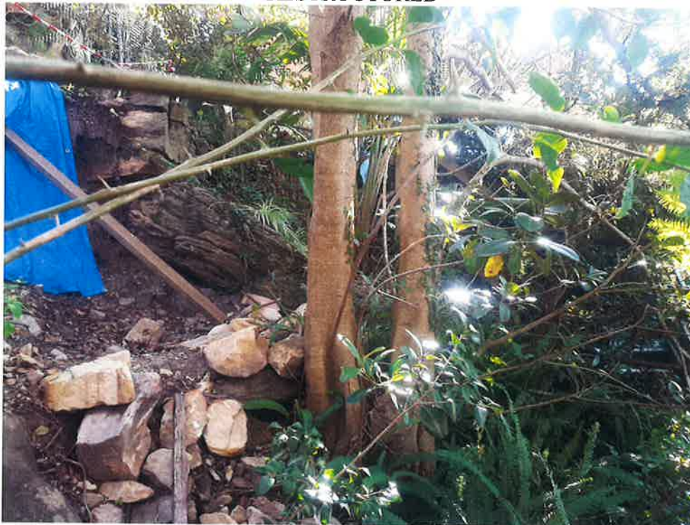
RETAINING TO BE REPLACED
